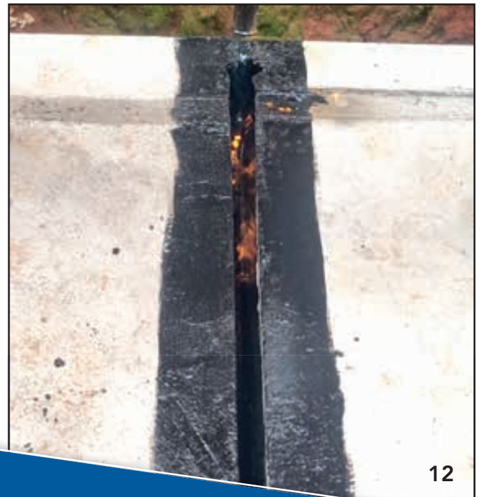
Denso Primer D™ & Denso™ Joint Sealer applied for all new concrete bases placed forward (external section).
