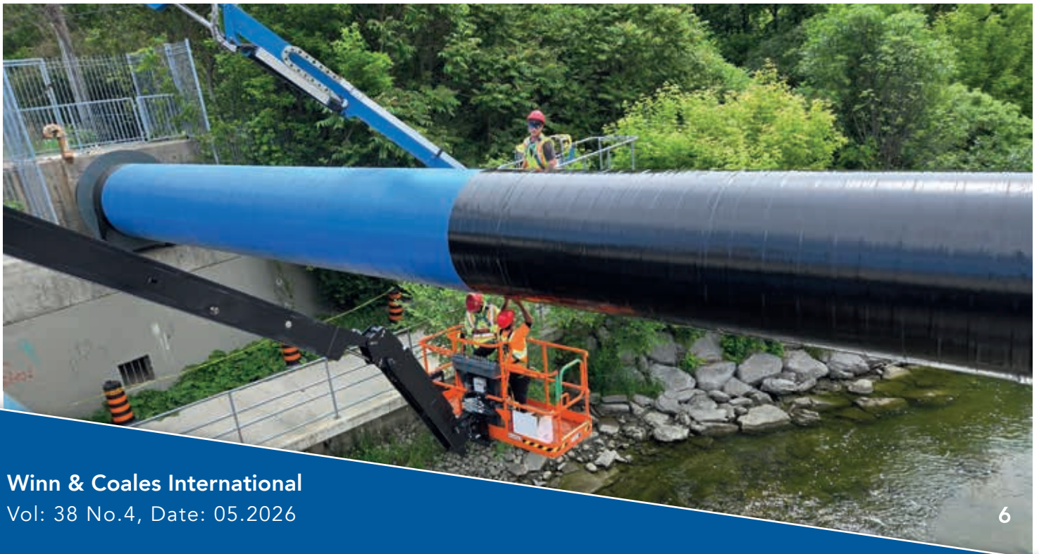
Below and top of page 9: A wrap of ViscoWrap™ ST (blue) is followed by a wrap of ViscoWrap™ PE (black).
