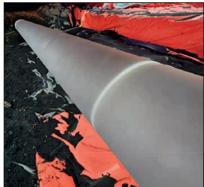
Below: All pipe surfaces were abrasive blast cleaned prior to applying the Protal 7200 liquid coating.
