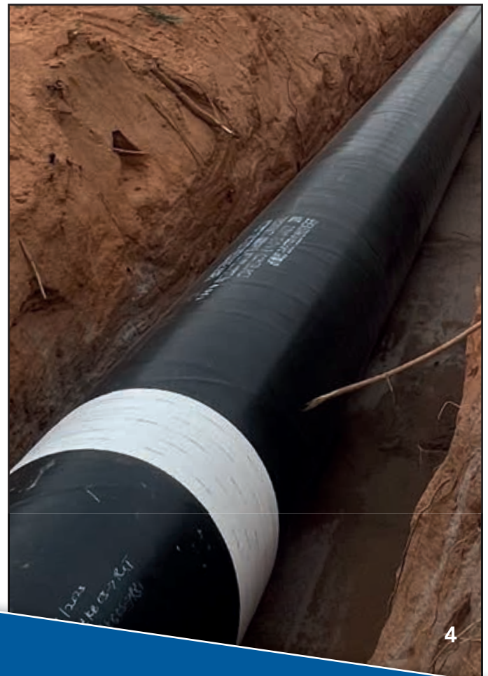
Below: Completed field joint wrapped with our Denso™ Liquid Field Joint Coating System.
