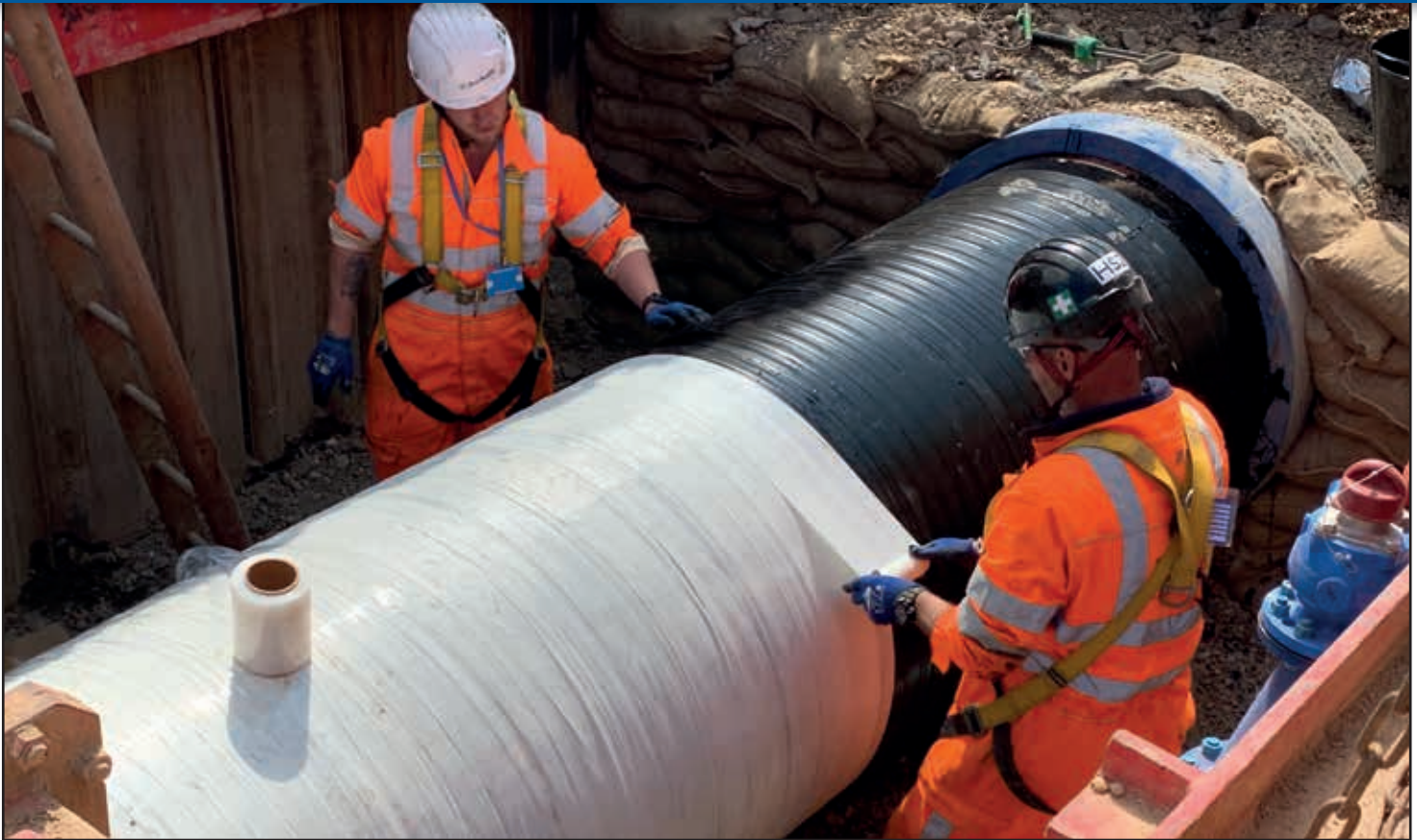
Above: Denso GOW is applied in a similar fashion, with a double layer of Denso Clear Outerwrap applied to aid curing and later removed.
