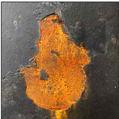
Example image showing tightly adhering corrosion prevention coating and corrosion (orange rust) that would not require removal.
