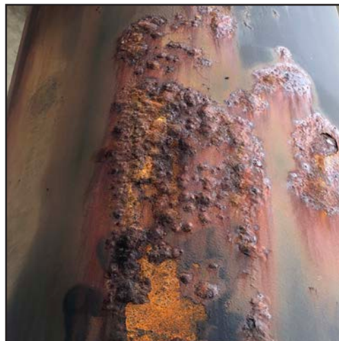
Example image of a pipe featuring a loosely adhering corrosion prevention coating that would require removal.
