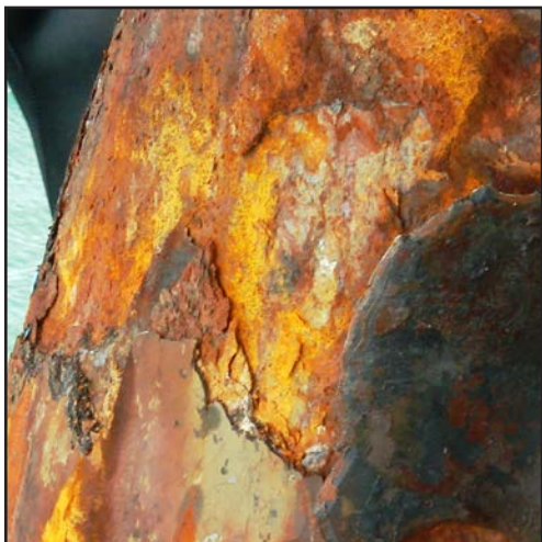
Example image of a pipe featuring loose corrosion that would require removal.
