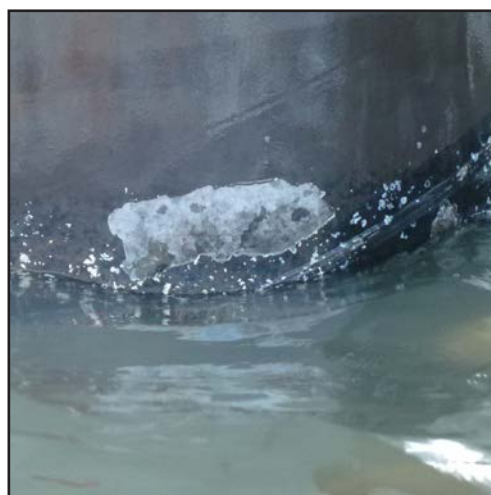
Example image of a pipe featuring acceptable levels of non-living, tightly adhering mineral deposits.
