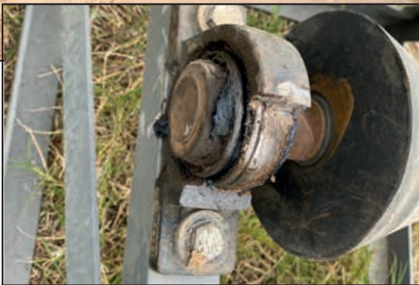
Failed pipe roller bearing.
