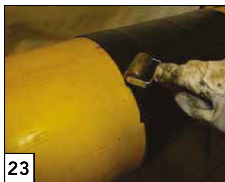
23 Roller the transition to the factory coating, the edge of the sleeve, the overlap of the sleeve and the area of the welded seam.
