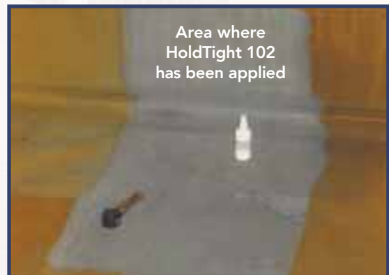
Above: View inside a tank where HoldTight 102 was applied to a panel. Note the flash rust that has appeared on the untreated area. The treated HoldTight 102 area will remain rust free for up to 48 hours or longer after application.
