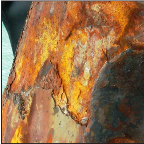
Example image of a pile featuring loose corrosion that would require removal.
